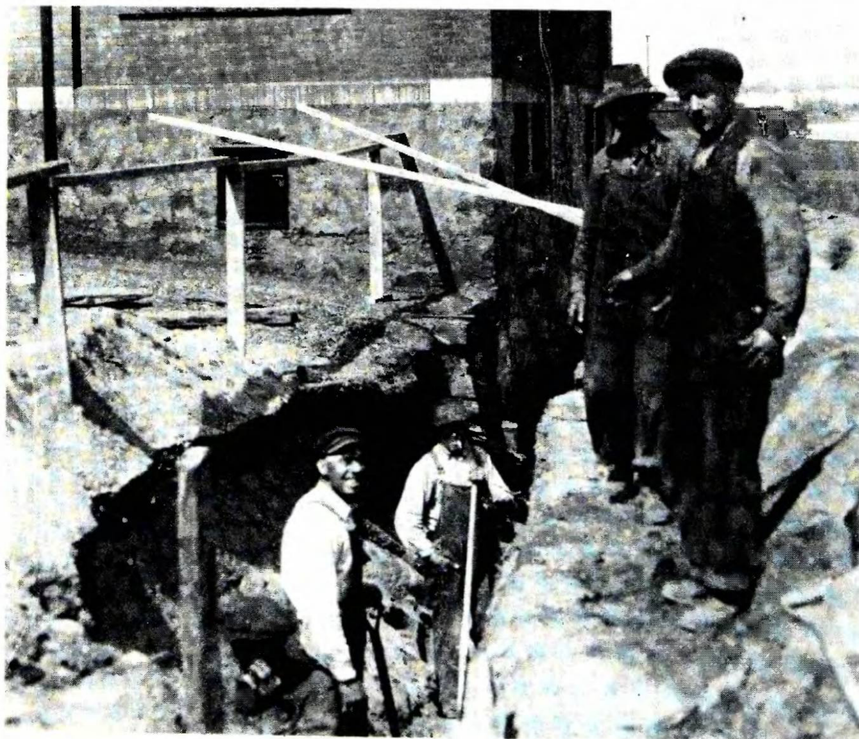
Below: Ukrainian workers laying sewer pipe, Port Arthur, Ontario, 1922. (Bobersky Collection, Oseredok, Winnipeg)
