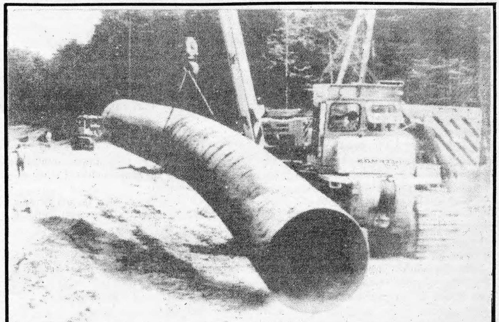
The Associated Press released this photo of construction work being done on the Ukrainian section of the Siberian pipeline. A Japanese tractor lifts West German pipe. In the summer of 1982 a great number of workers and specialists from East Germany were brought in to work on the pipeline on Ukrainian territory.
